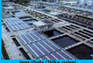
Japan/Osaka (360kw system)
