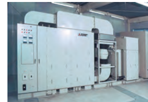
Mitsubishi Electric photovoltaic inverter (400kW, installed in 1985)
